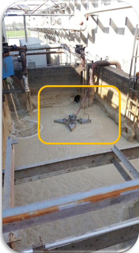
Floating AutoWeir skimming solids in EQ Tank
