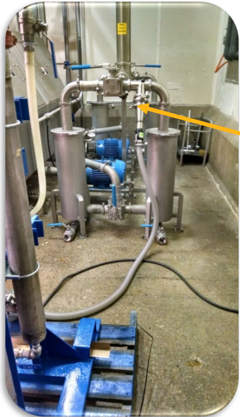
Pilot connection to existing Rocket Filter
