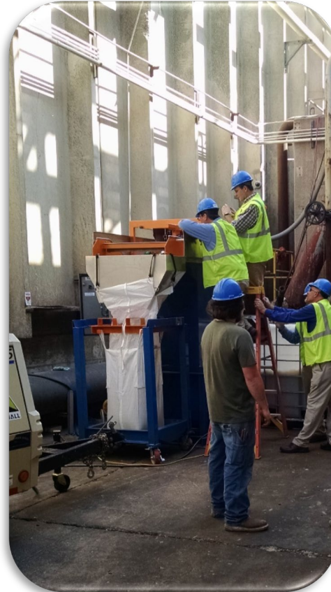
Dewatering Bag System next to EQ Tank
